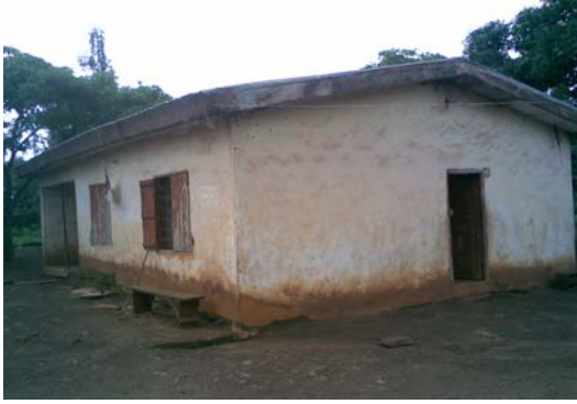
Before: Dilapidated Health Facility
